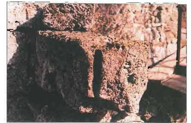
95 Frankopanska kula, zapadno pročelje, ostatak prozorskog okvira na trećem katu Frankopan Tower, western façade, remains of the window frame in the third floor
